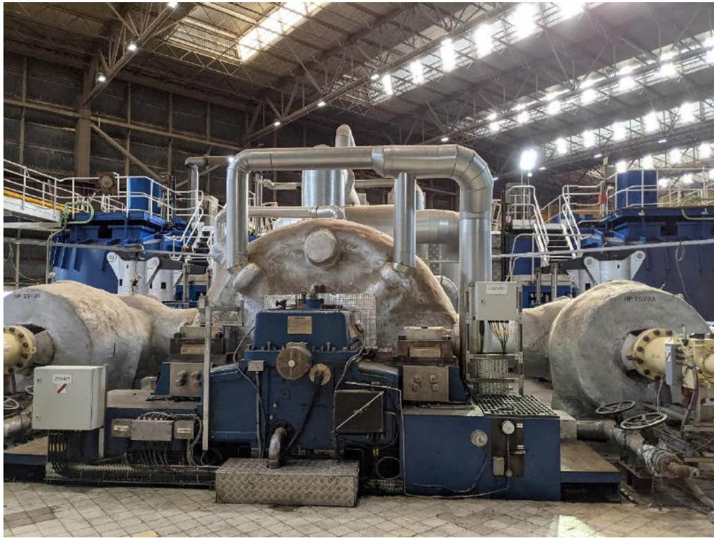
Photo 3: View of turbines within the turbine hall. The turbine hall is located in the centre of the Drax Power Station Site.
