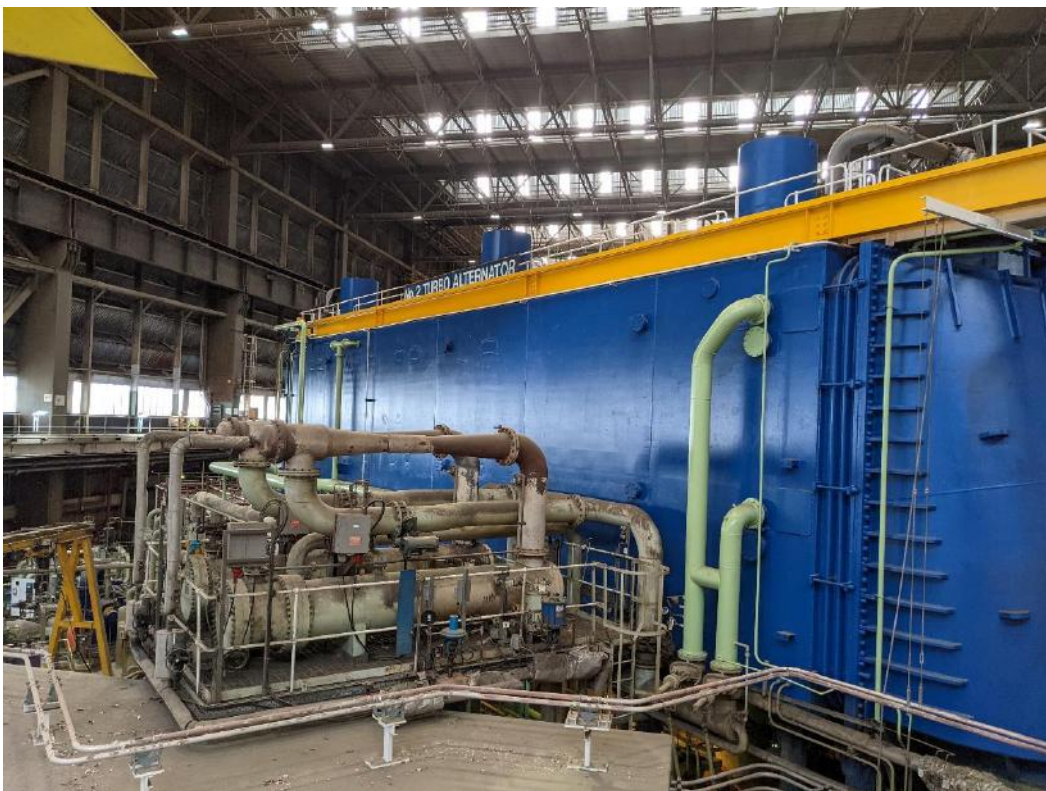
Photo 4: View of condenser units within the turbine hall.
